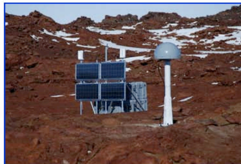
Permanent GPS station BURI at Butcher Ridge, Antarctica. POLENET GPS station BURI at Butcher Ridge in the Transantarctic Mountains features wind and solar power, and Iridium communications for year-round autonomous operation. This station was installed by UNAVCO for Land Information New Zealand, and is part of the New Zealand contribution to the international POLENET project. A goal of the POLENET project is using bedrock geodesy to constrain past and present day changes in Antarctica's ice mass.
