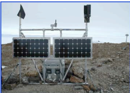
GPS Prototype Station MIN0 at Minna Bluff, Antarctica. First prototype station deployed under UNAVCO/PASSCAL Remote Stations MRI project. A moderately sized battery bank with charging from solar and wind provided nearly continuous year-round operation and communications during 2007.
