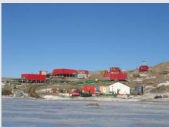
Overview of the new Troll station still under construction (Photo: Stein Tronstad, Norwegian Polar Institute)
